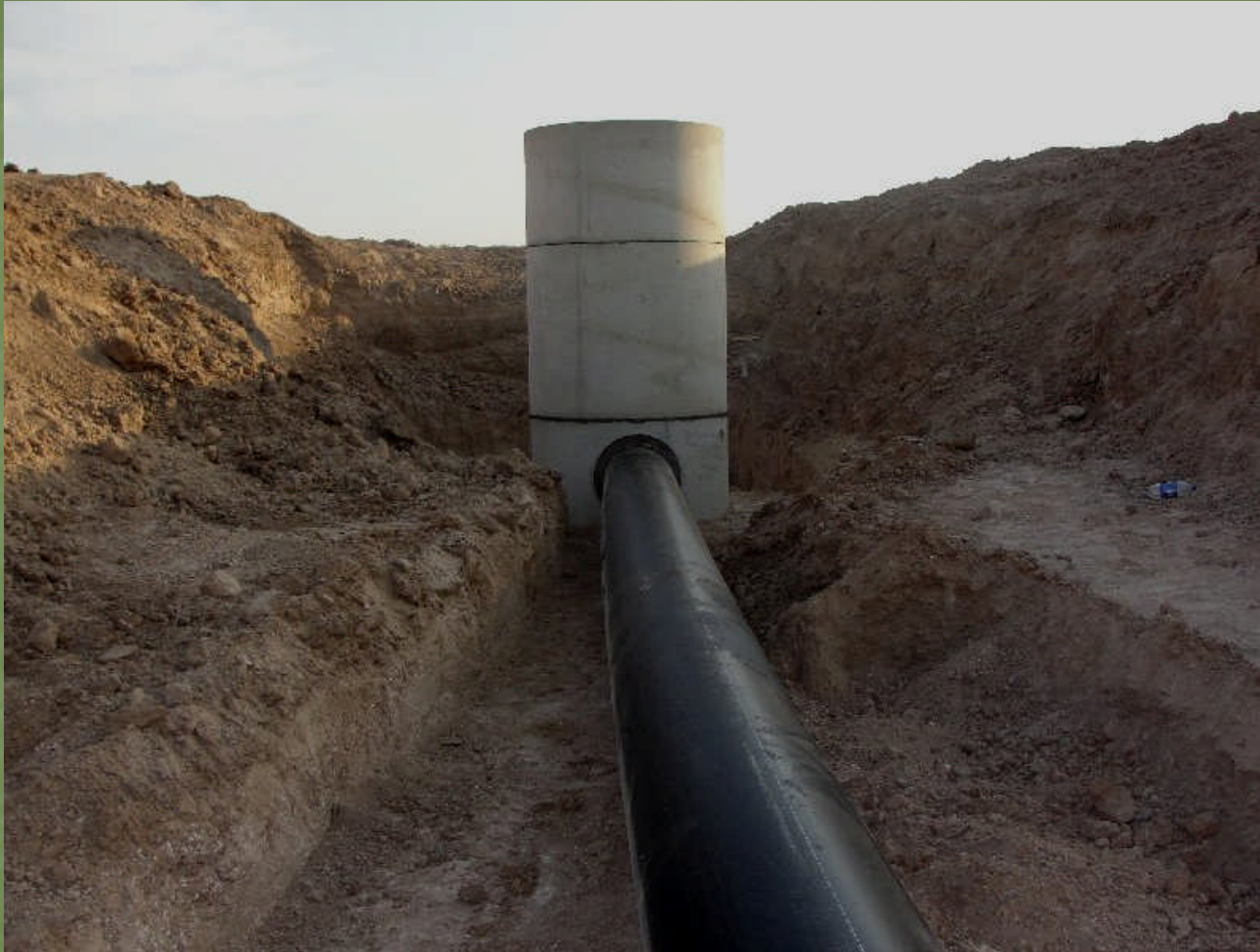
Irrigation Wet-well Intake Pipe
