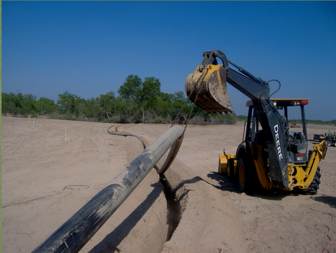
HDPE Irrigation Mainline
